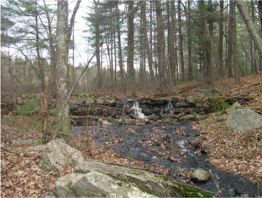
Photo 5 – Dean Pond Dam and spillway, downstream side (11/2010, photo by Shary Page Berg)
