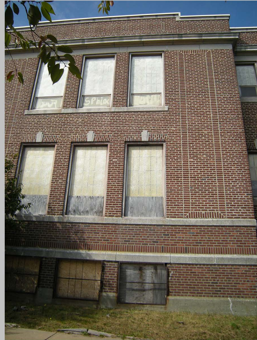
14. Brick panel at right, and above windows in parapet, beltcourses in cast stone and brick soldier course
