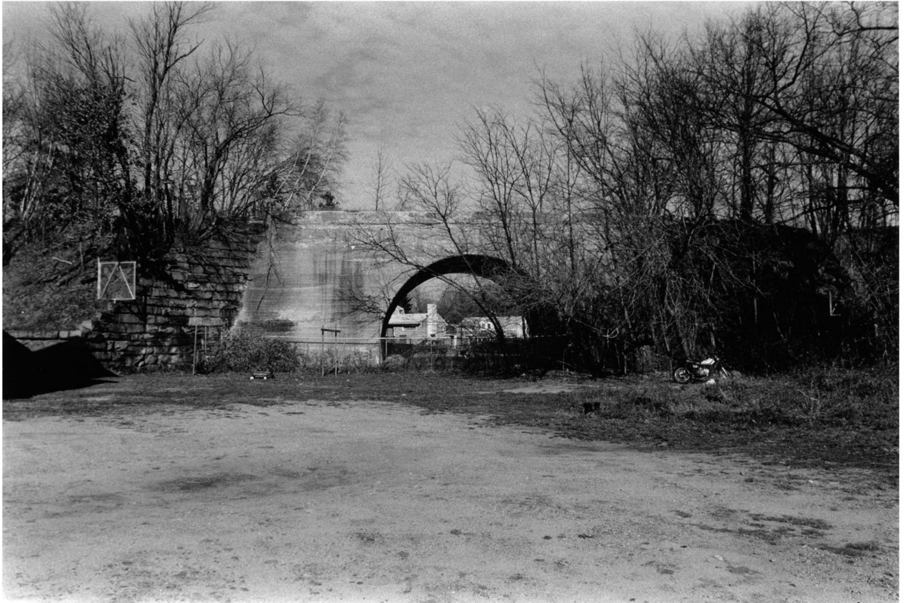
4. View looking north showing, from left to right, West Embankment, Single-Arch Bridge West Abutment, Single-Arch Bridge, Single-Arch Bridge East Abutment, and Middle Embankment (Photographer: Matthew A. Kierstead, 18 November 1999)
