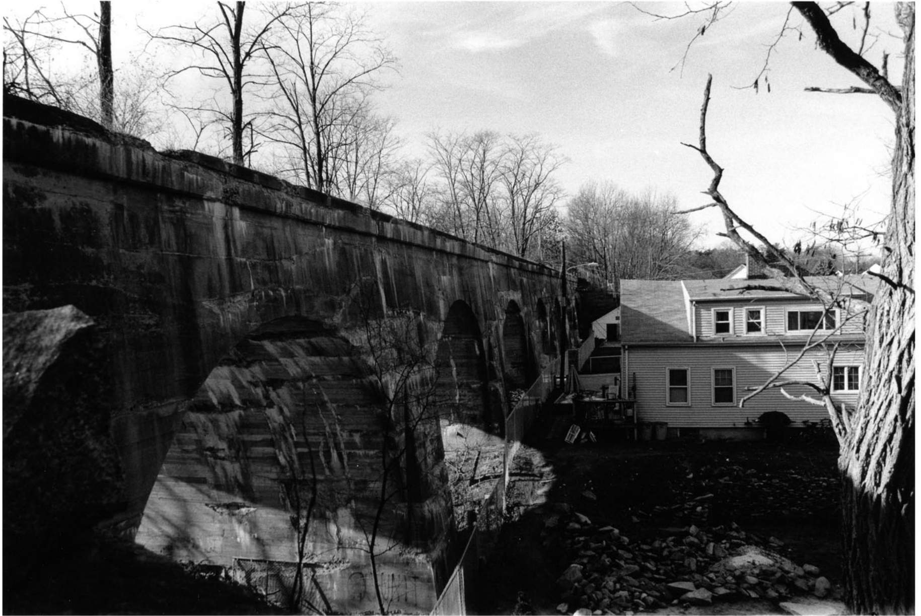
2. View looking west showing north face of Multiple-Arch Bridge with Waterford mill housing at right (Photographer: Matthew A. Kierstead, 18 November 1999)
